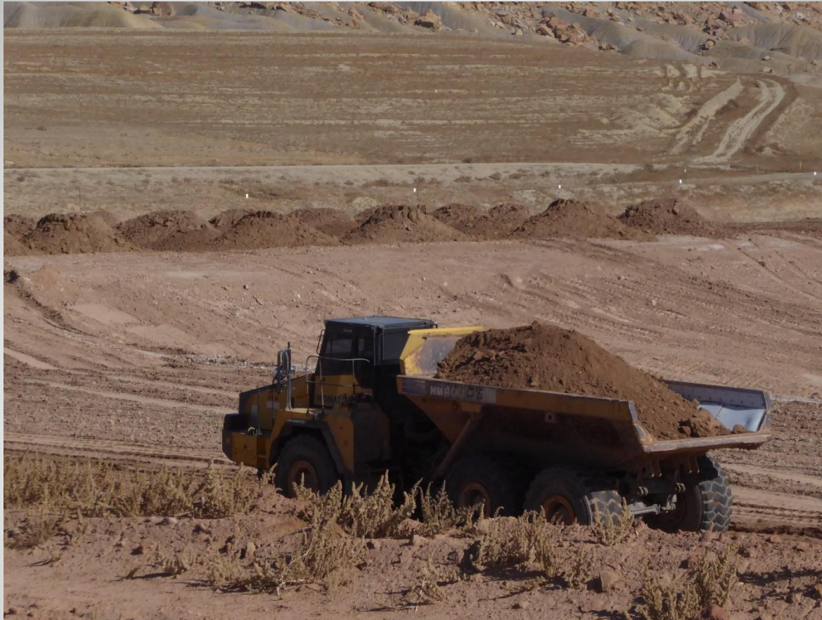
Transporting RRM to another compaction Area. Note massive surface water flow protection wedge in background above cell. Note access road to the top of wedge shown in the upper right for scale.
